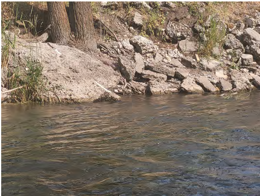
Photo 2 Degraded riverbank and riparian zone in API for Alternative 1 (north of the river alternative), contributing to cumulative impacts to the Logan River.
